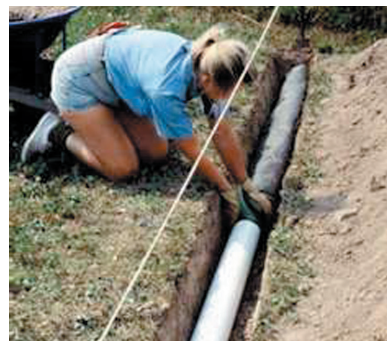
Figure 280: Underground Refrigerant Piping.
