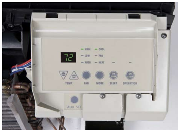
Enclosure cover removed.
