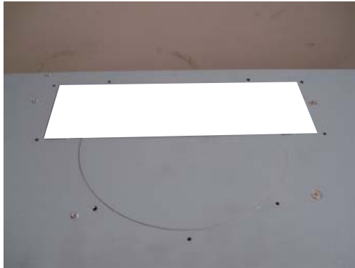
Vertical Ducting (3-1/4"x10" Rectangular)
